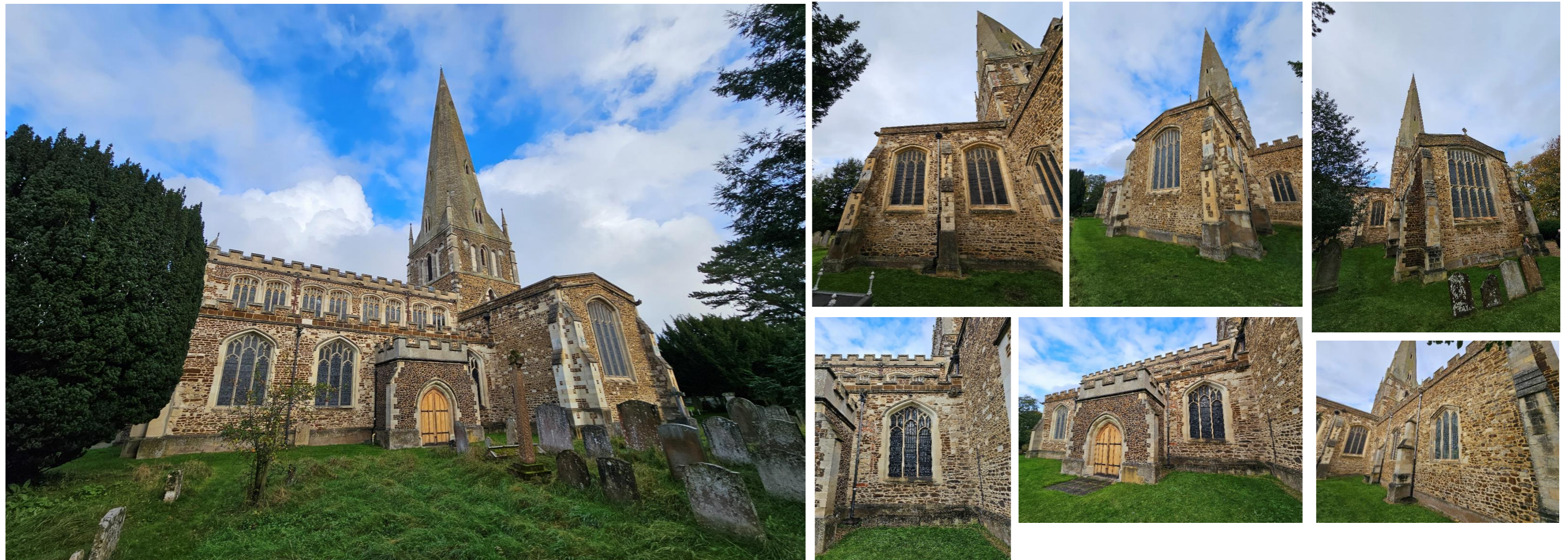
Figure 910 10 - South and East Elevation. Note the grandiose Clerestory and windows are all in Perpendicular style. Note again that buttresses have been substantially repaired, tower heightened and altered with Gothic Revival pediments. Original roof form above south Transept and no battlement. new ones on the south porch (also compact nature of the material).
